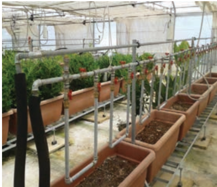
Figure 3. The cooling pipes inside the greenhouse.
