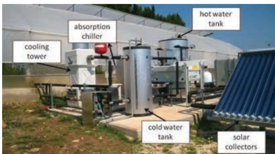
Figure 2. The solar cooling system at the experimental center of the University of Bari, Valenzano (Bari, Italy).
