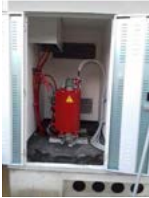
Figure 5. MV/LV substation with a single 400 kVA transformer.
