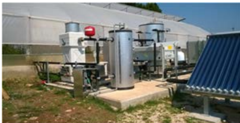
Figure 2. The experimental solar cooling plant.
