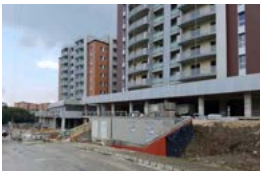
Figure 4. Picture of the case study building under construction, with a private MV/LV substation.
